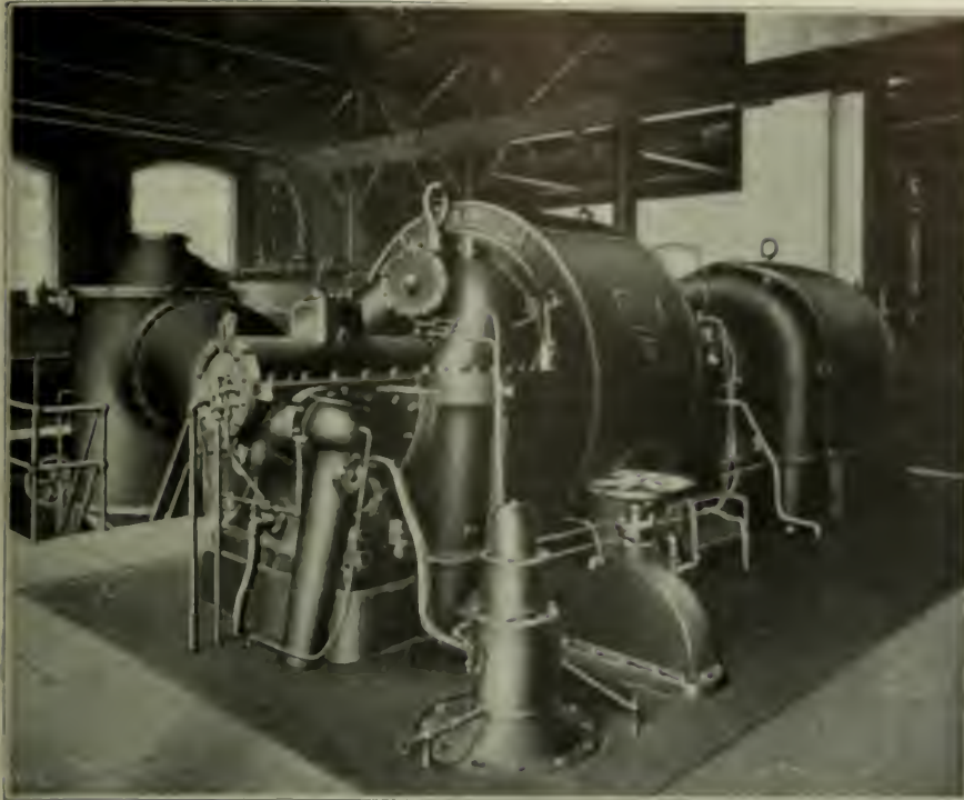
FIG. 4. LOW-PRESSURE TURBINE WITH THROTTLE VALVE IN FOREGROUND
